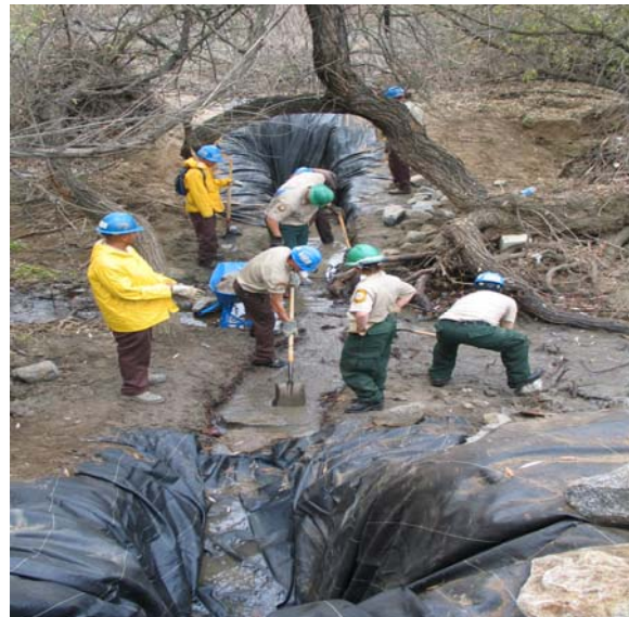
Site of grade stabilizer before installation of keyway. Over 10,000 pounds of rock were placed by hand by crews from the California Conservation Corps to complete the project. Work on the stabilizer began in winter of 2005.
