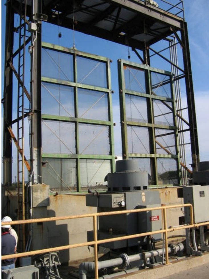
Figure B4-1. Unit 1 slide screens. Unit 2 screens are identical.
