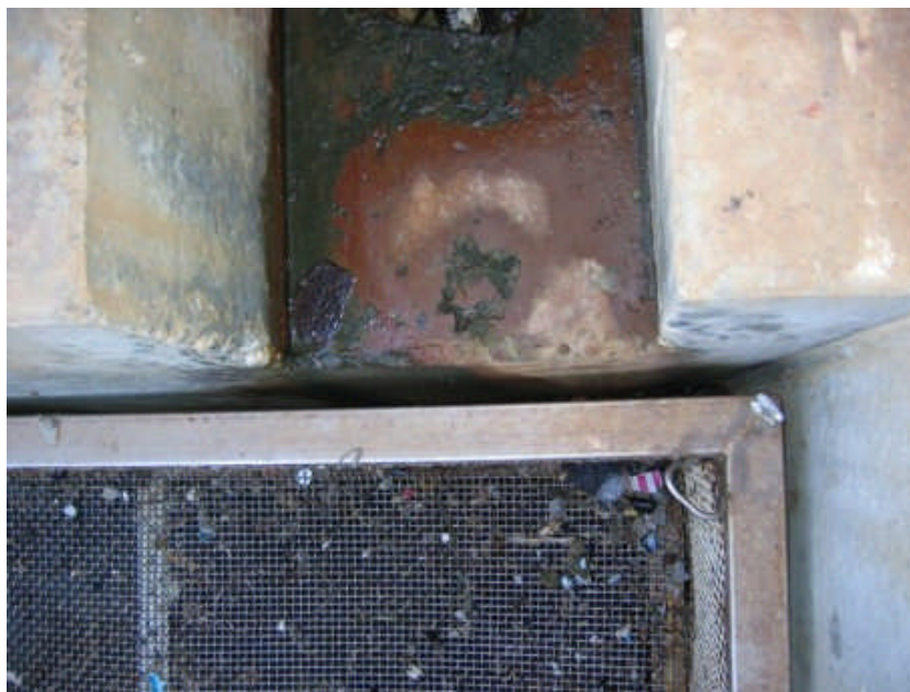
Figure B4-2. Sump basket at Unit 2 (top). Unit 1 is identical. Note the space between the trough and the edge of the sump basket (bottom).
