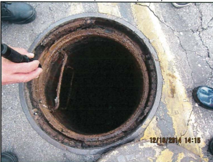
Photo 5: Manhole and sewer line inspection; note manhole ring corrosion
