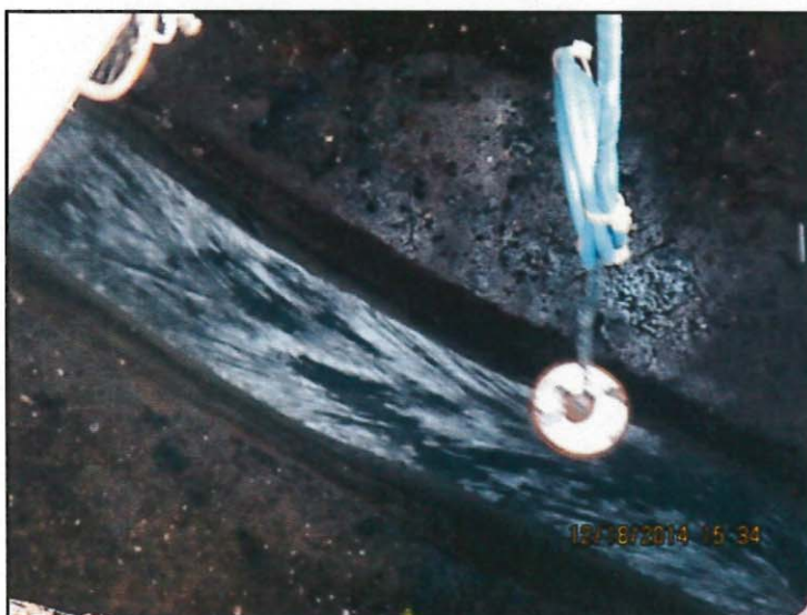
Photo 29: "Smart Cover" ultrasonic sensor (view 1)
