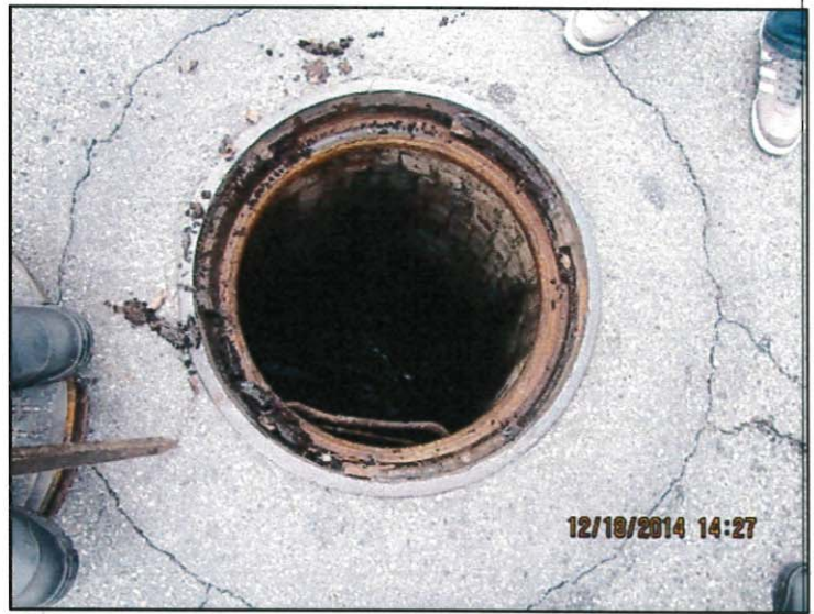
Photo 8: Manhole and sewer line inspection; note manhole ring corrosion
