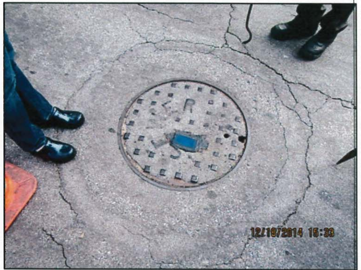
Photo 26: "Smart Cover" inspection site (view 2)
