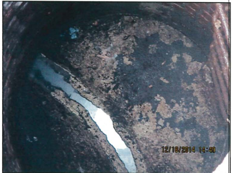
Photo 18: Manhole inspection (view 3): note heavy FOG buildup on manhole base and in sewer line
