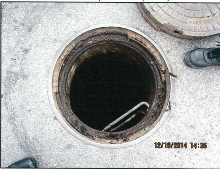
Photo 13: Manhole and sewer line inspection; note manhole ring corrosion
