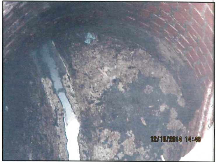
Photo 16: Manhole inspection (view 1): note heavy FOG buildup on manhole base and in sewer line
