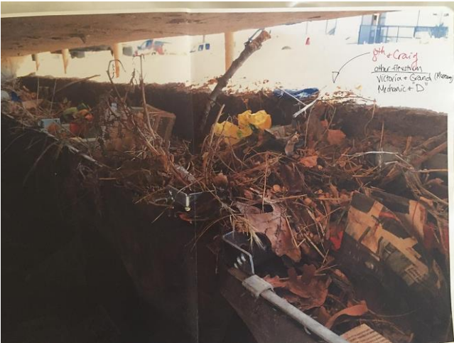
Photo 6: Improperly maintained Open Throat Curb Inlet Filter in Pueblo, Colorado.
