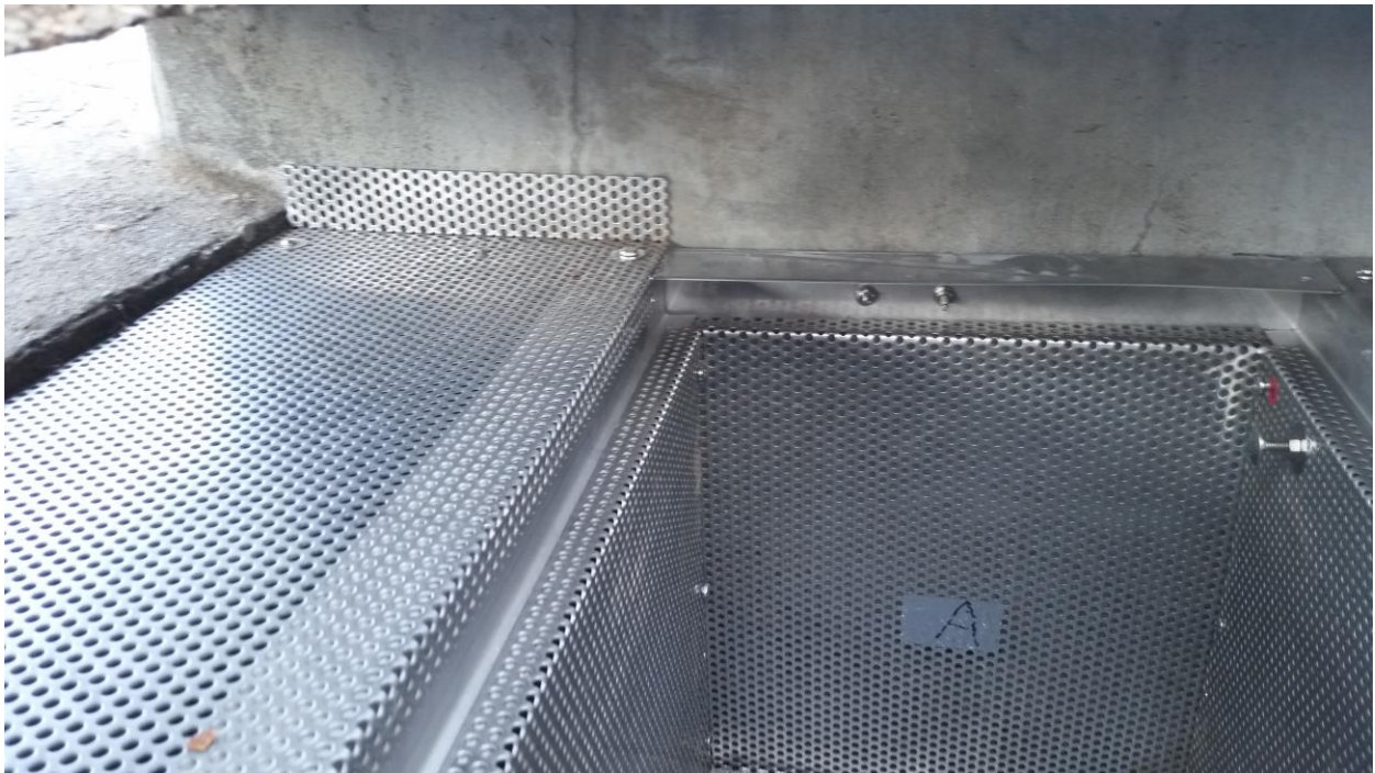
Figure 3. Installed Curb Inlet insert 100% collection at front vault wall
