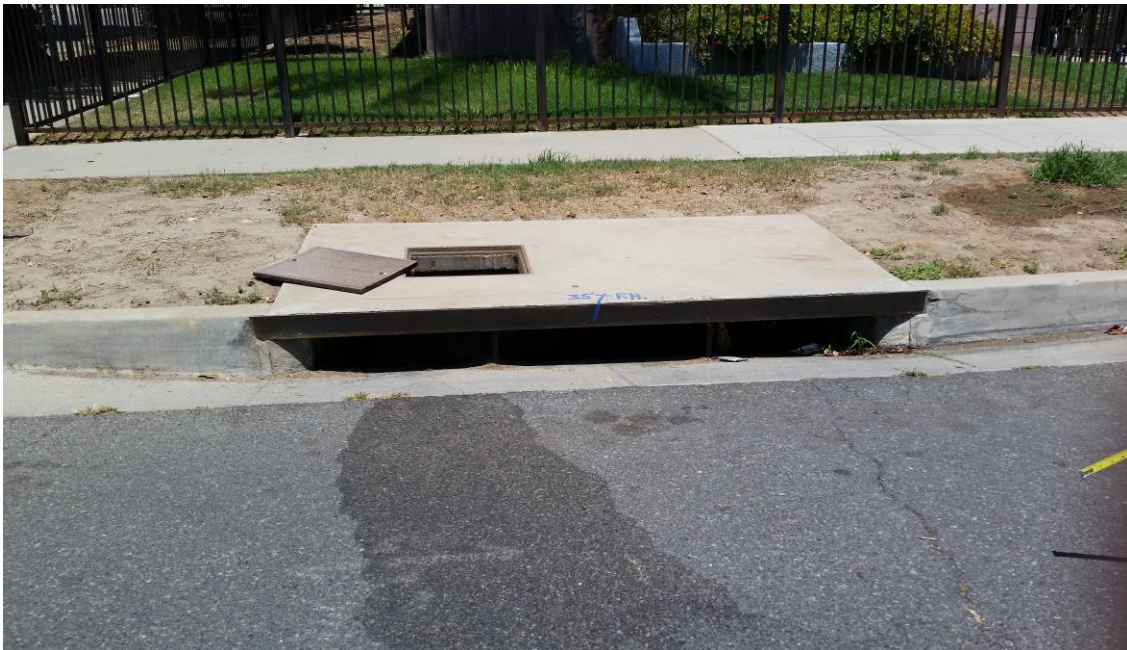
Figure 1. Cleaned curb inlet for CleanWay's Curb Inlet filtration insert
