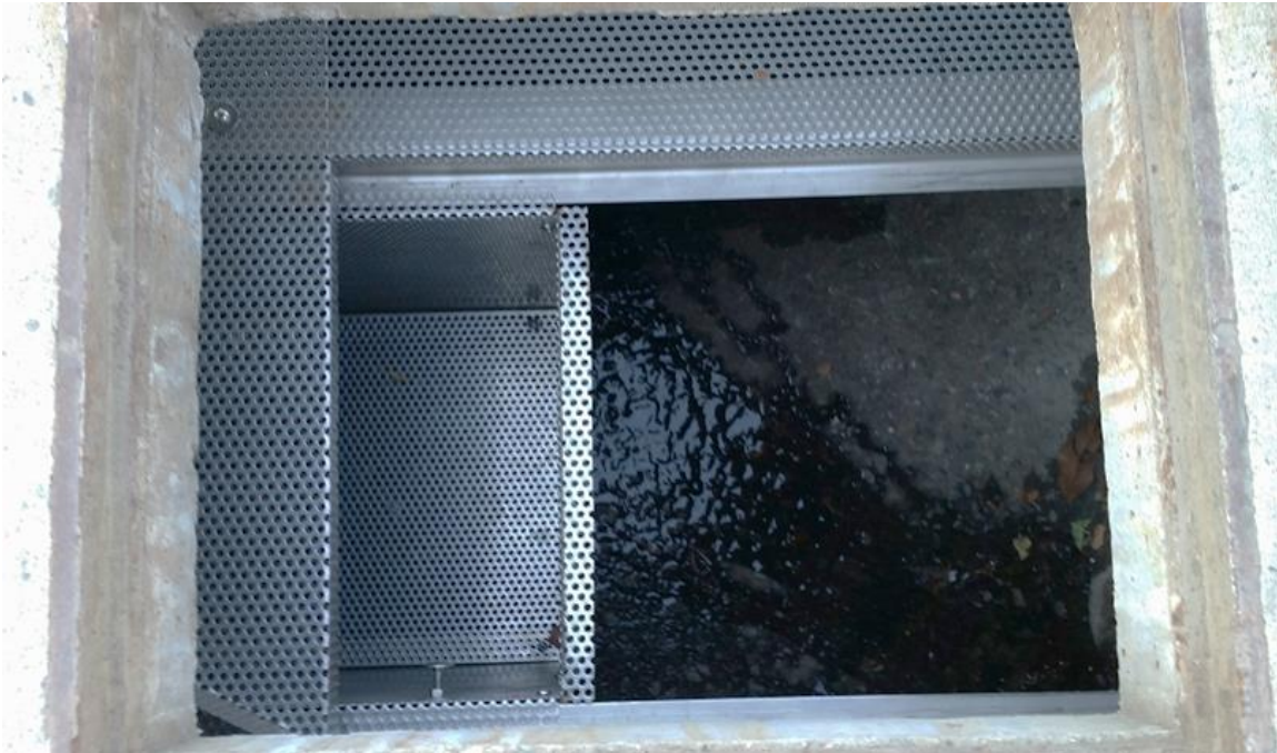
Figure 7. Curb Inlet vector control point of access underneath sliding collection basket
