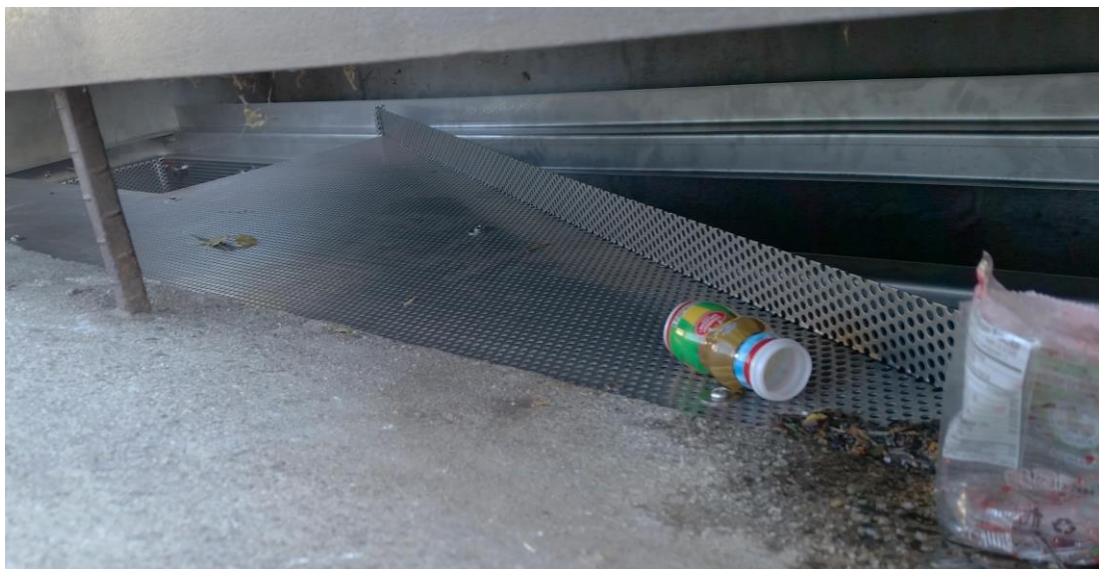
Figure 8. Curb Inlet vector control point of access behind unit lip on end opposite of collection basket
