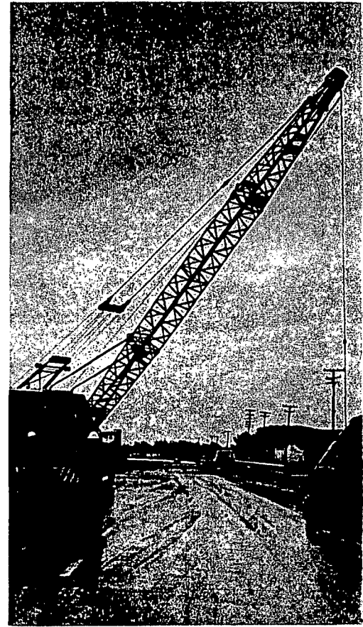
Crane removes logs washed up on undamaged section of county road near Ferndale in order to use it for detour for Redwood Highway.
