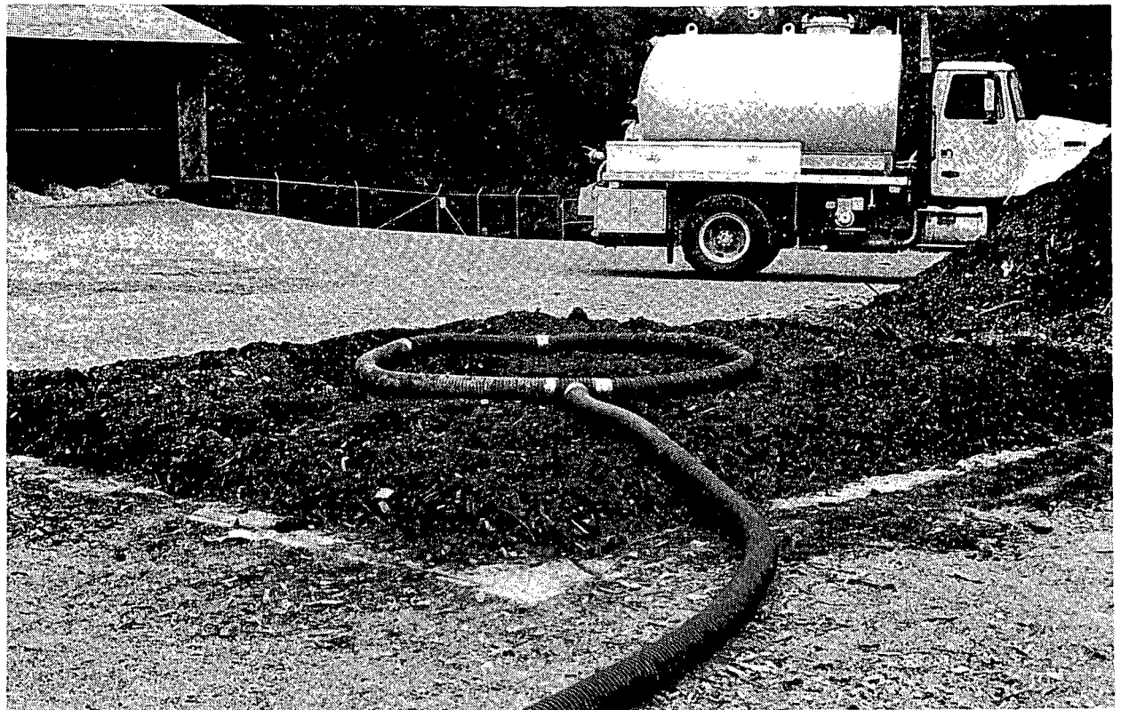
Figure 6: A loop of four inch perforated pipe is laid in the center of the mattress.
