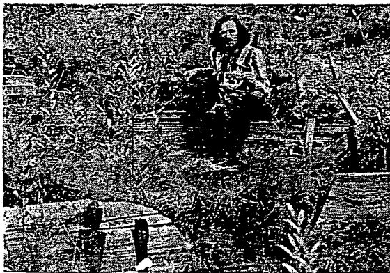
FIGURE 8. After one season the catch basins upstream of each check dam are filled with sediment. Sprouting willow stem cuttings and other plants are beginning to stabilise channel banks and bed.
