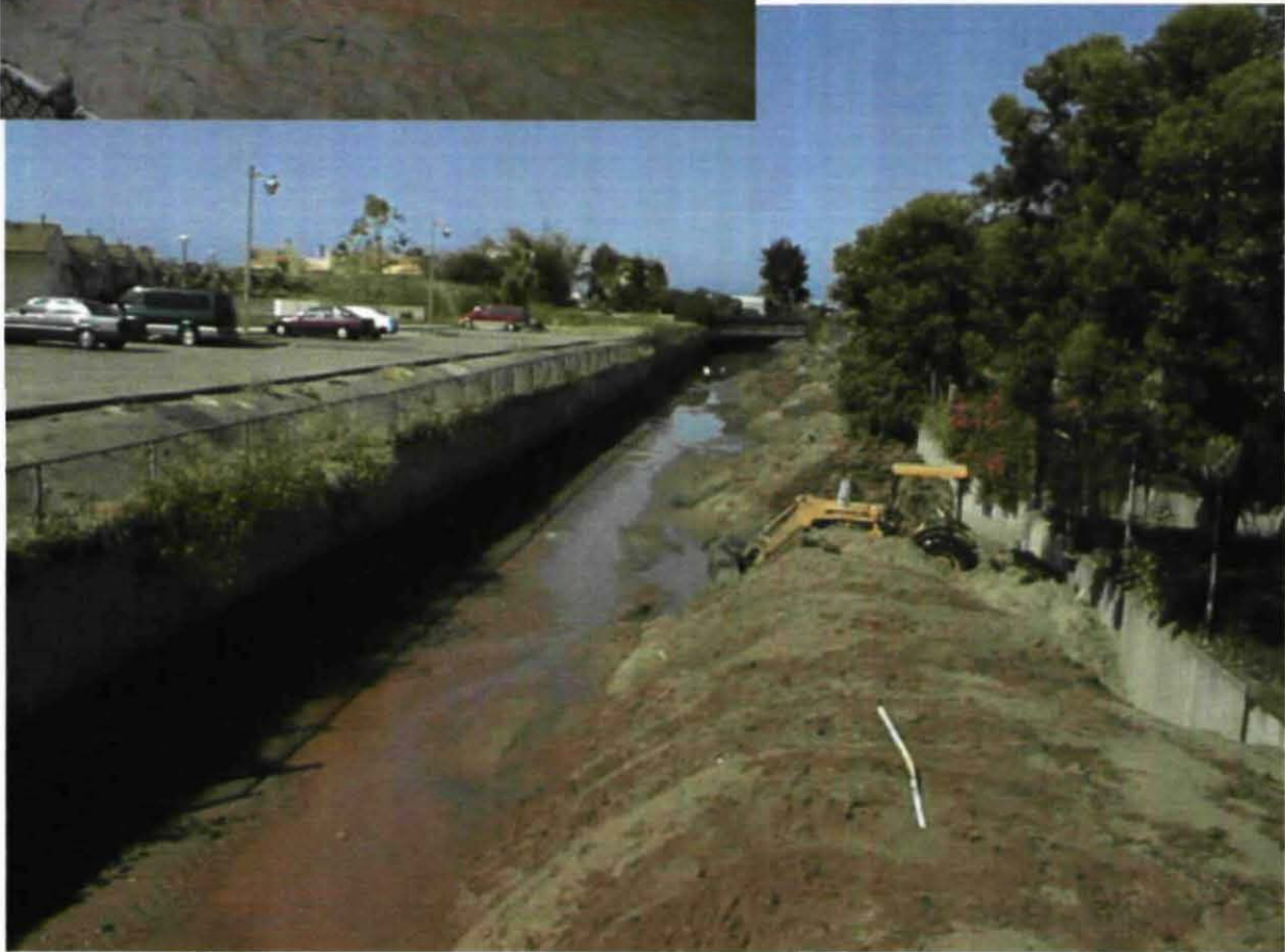
Figure 6. The upper photo shows sediment-laden storm flow in Franklin Creek during a storm on March 15, 2003. Sediment concentrations ranged up to 10 g/L during this event. The lower photo shows channel cleaning operations in Franklin Creek in April 2001 following the large storm of March 3-4, 2001. This is the sediment from a single large event. Deposited sediment volumes from large storms are almost unread, demonstrating a substantial and ongoing sedimentation problem for the Carpinteria Salt Marsh (the main tributaries of which are Franklin and Santa Monica creeks).
