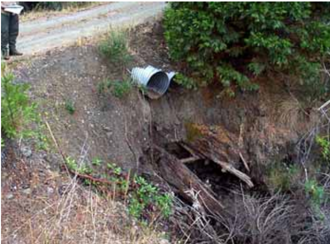
Figure 36. Watercourse crossing at high risk of failing.
