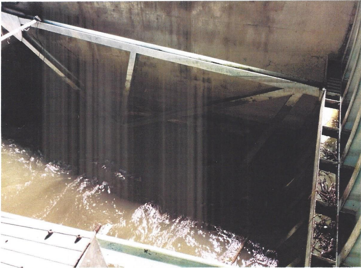
Photo 3 – Large log caught in radial gate arm.
