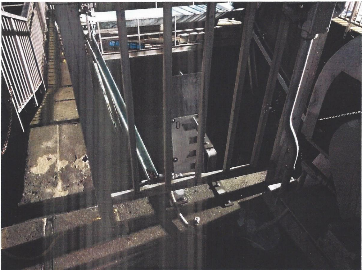
Photo 4 – Staff gauge on end of radial gate (typical).
