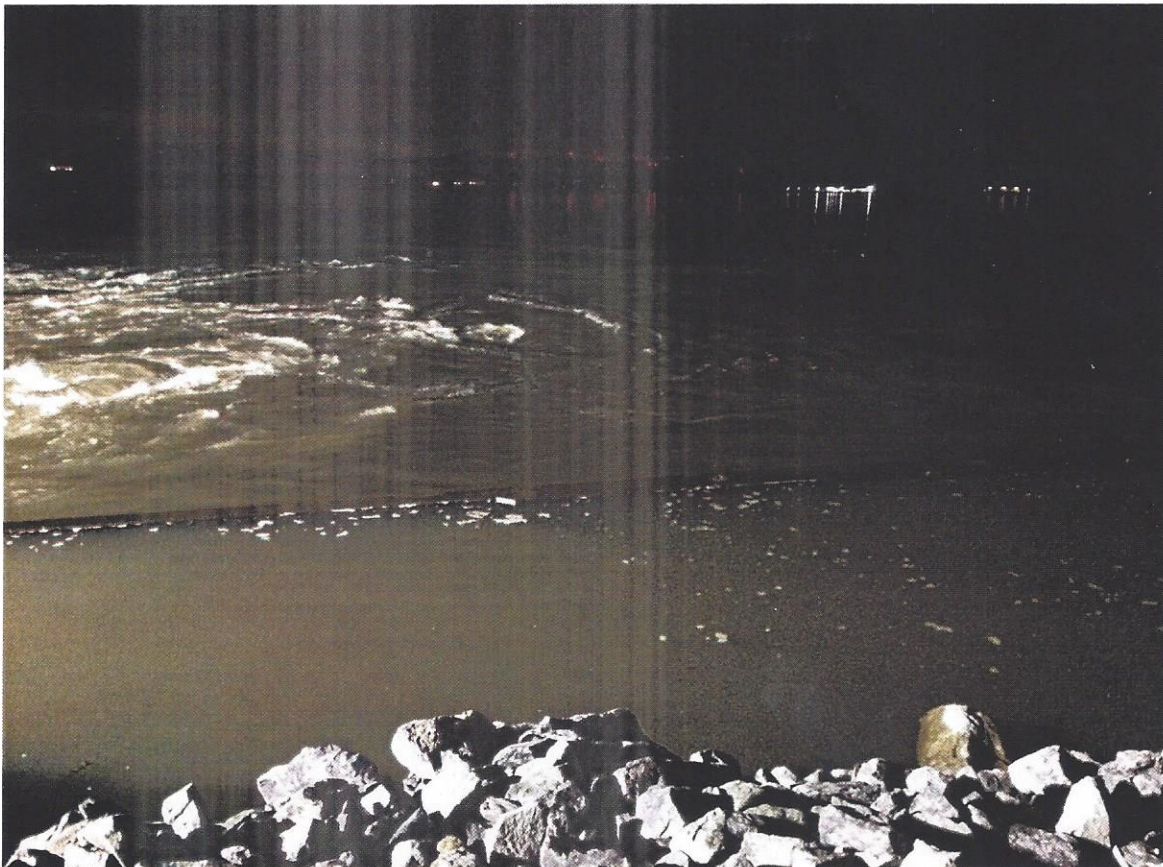
Photo 2 – View of D/S right wing wall repair and surface turbulence.
