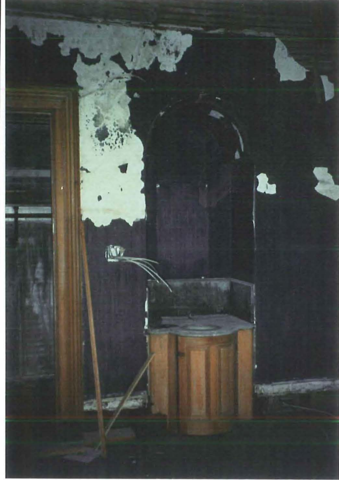
Damage to Master Bedroom
