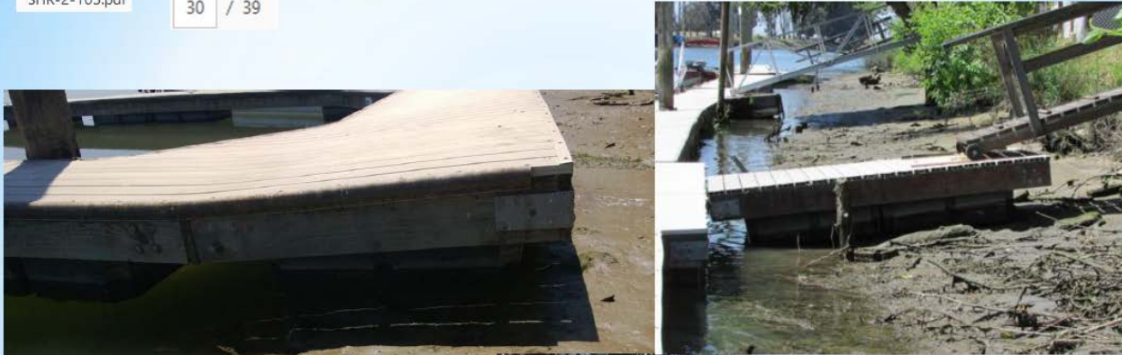
Bending of the bolts to break and to crack at mud
