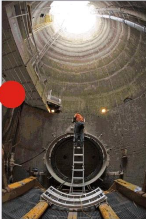
The pit for the tunnel under the river is readied for the boring machine.
