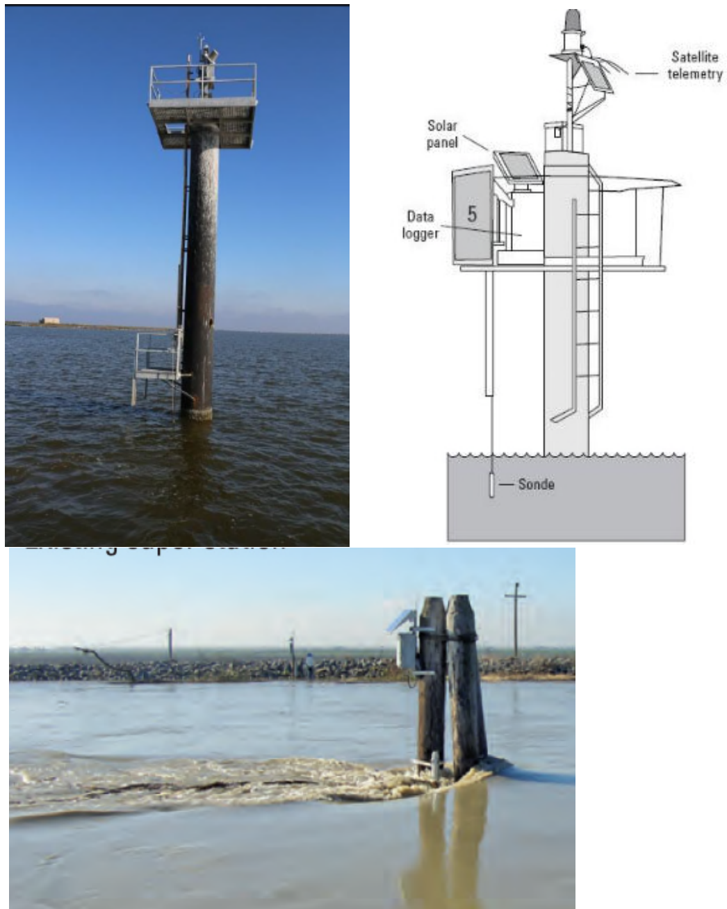
Figure C-1. Examples of Pier Mounted Monitoring Stations
