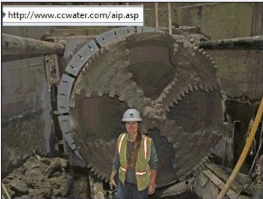
CCWD Senior Engineer Rachel Martin stands in front of the boring machine as it completed its journey under Old River.
