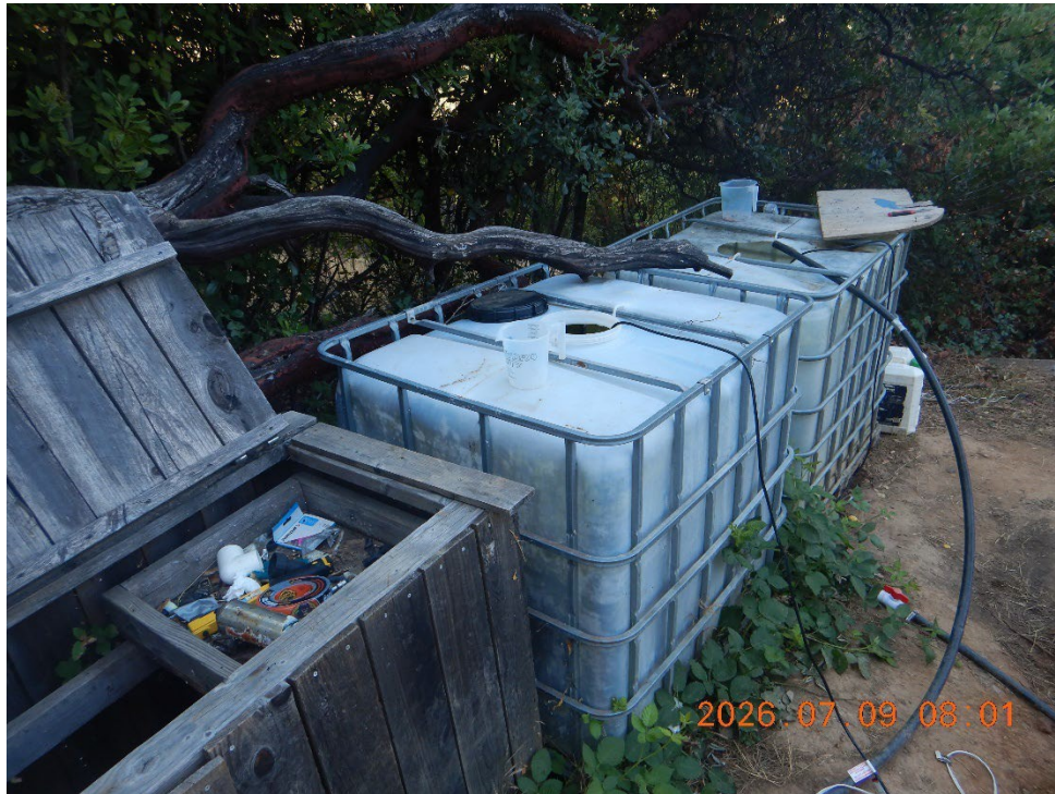
Photo 1 (POS2): Tanks 2 and 3 without lids or overflow protection.
