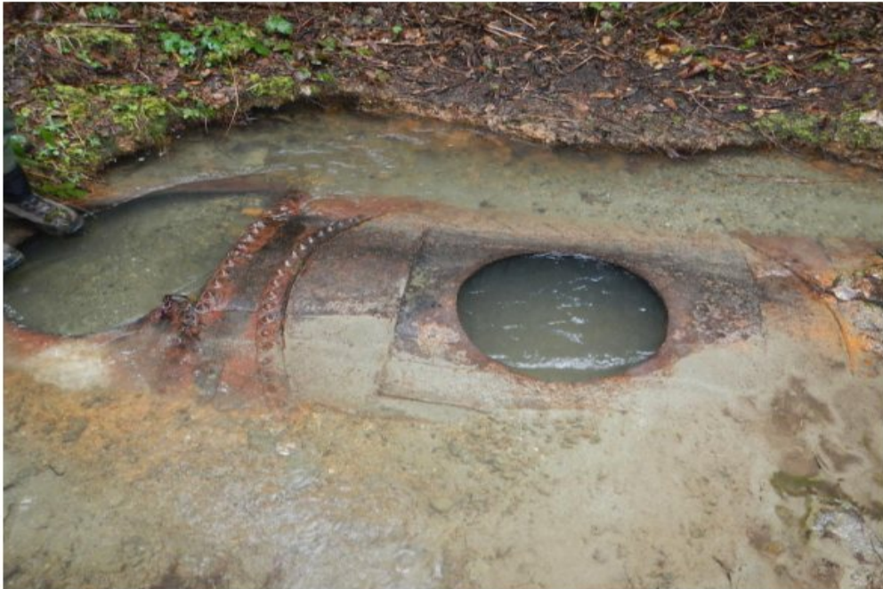
Figure 6. Failed Sediment Trap
