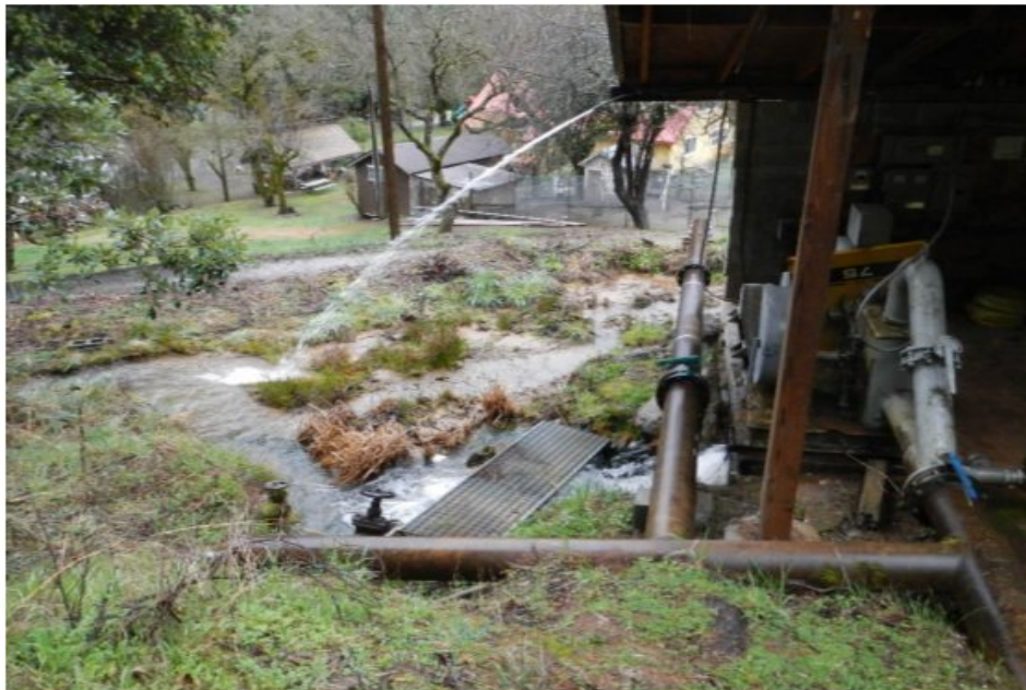
Figure 2. Outflow from MMR Hydroplant
