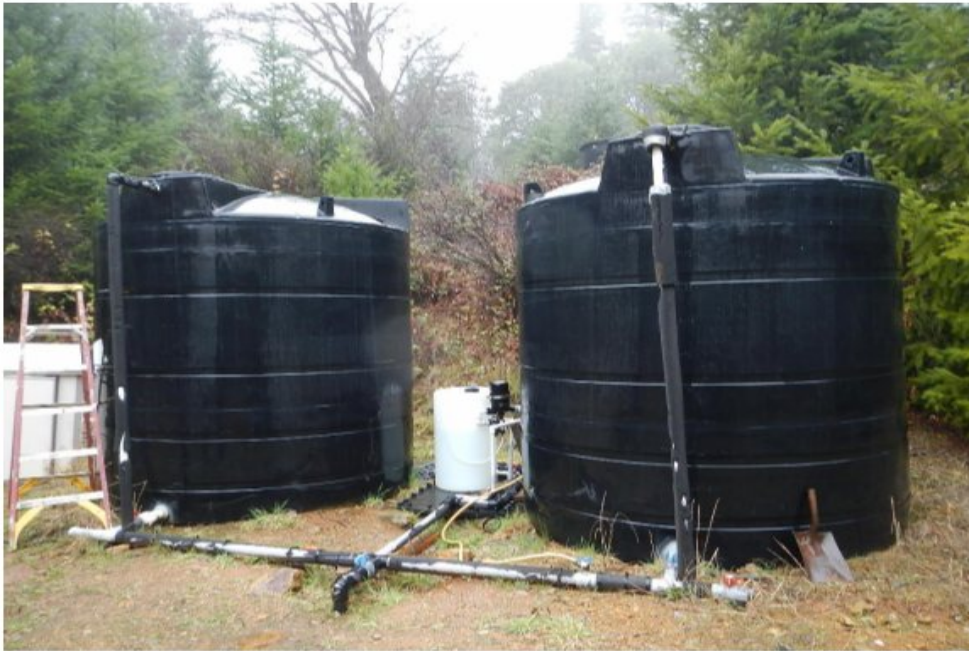
Figure 3. Domestic water treatment facility
