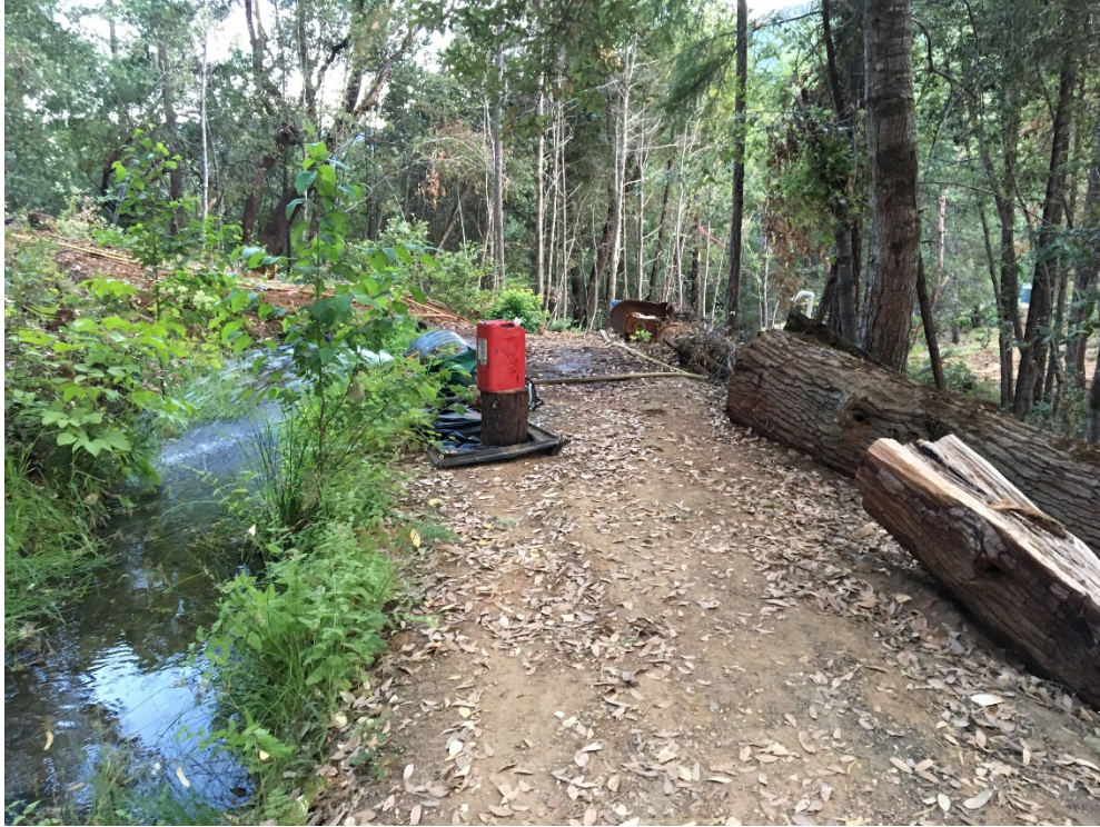
Exhibit MMR-10 Photograph #4 A pump is set up to pump water from the diversion to fill fire engines for fire suppression efforts.
