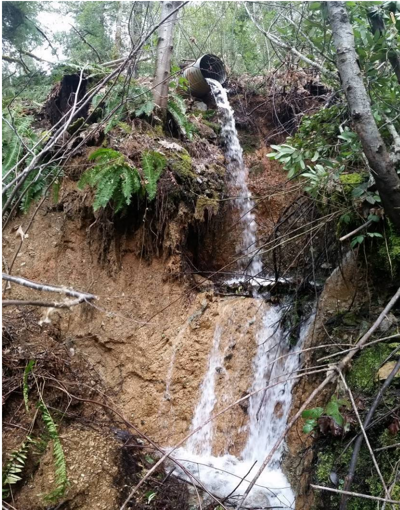
Figure 3. Upstream view of the shotgun culvert located at an unnamed tributary to Stanshaw Creek, Station 474.
