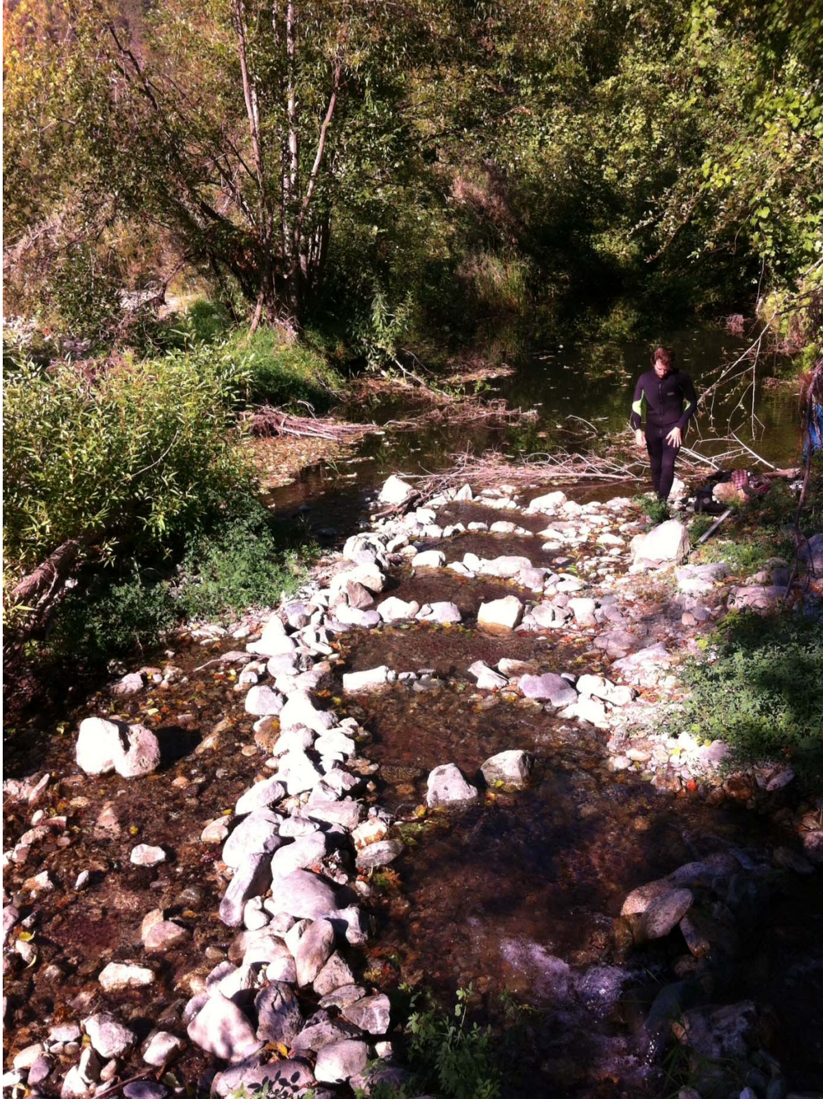
Photo 3. Downstream view of second berm-lined channel directing portion of Stanshaw Creek flow to the floodplain pond. The pond outflow, obscured by bushes, is to the left.
