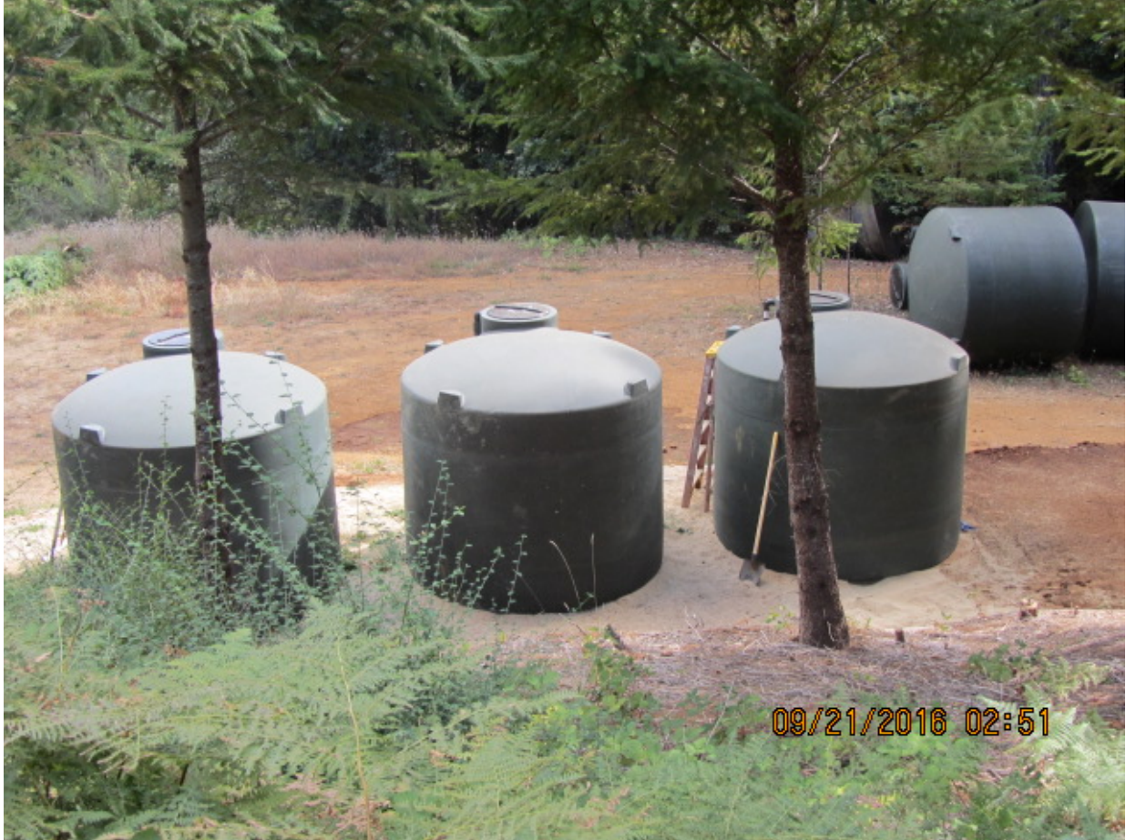
Exhibit MMR-03 Photograph #4 – Five of the seven water storage tanks at the Ranch during installation
