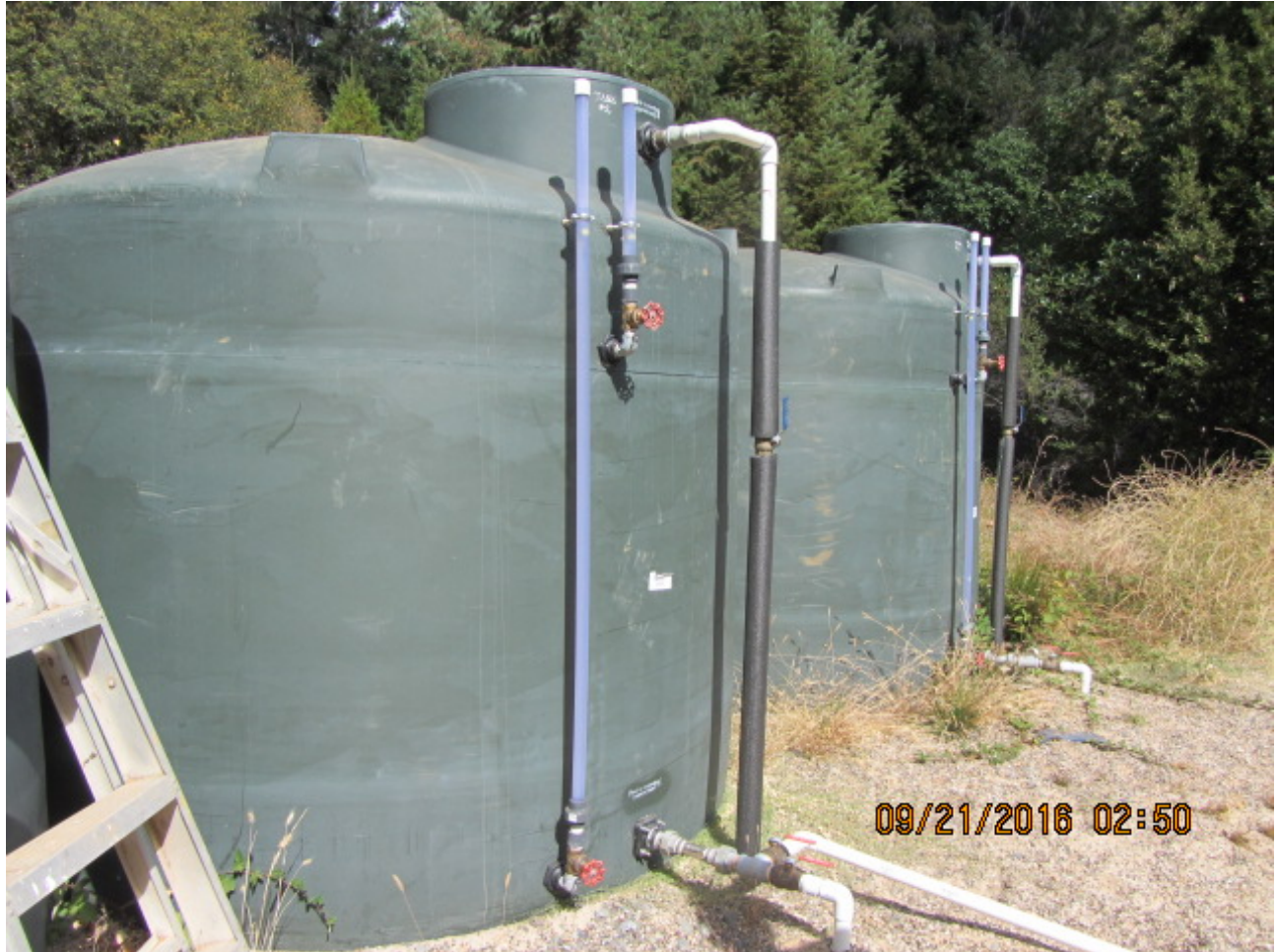
Exhibit MMR-03 Photograph #1 – Water treatment and storage tanks for domestic and consumptive use water
