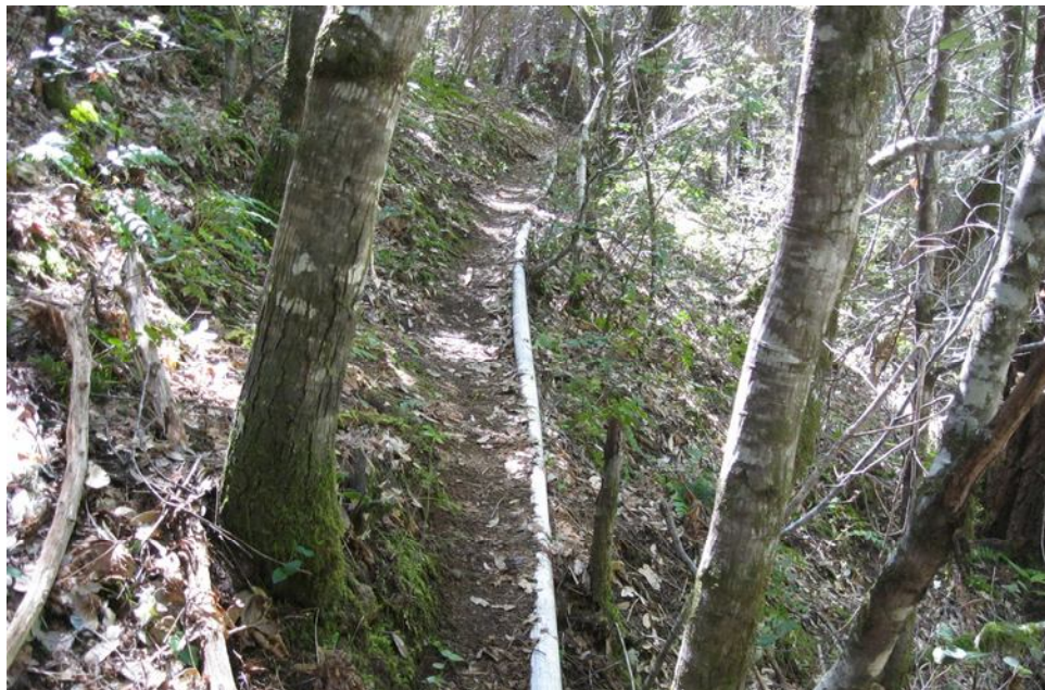
Photo 9 - 3-inch pipeline transporting water from POD # 1
