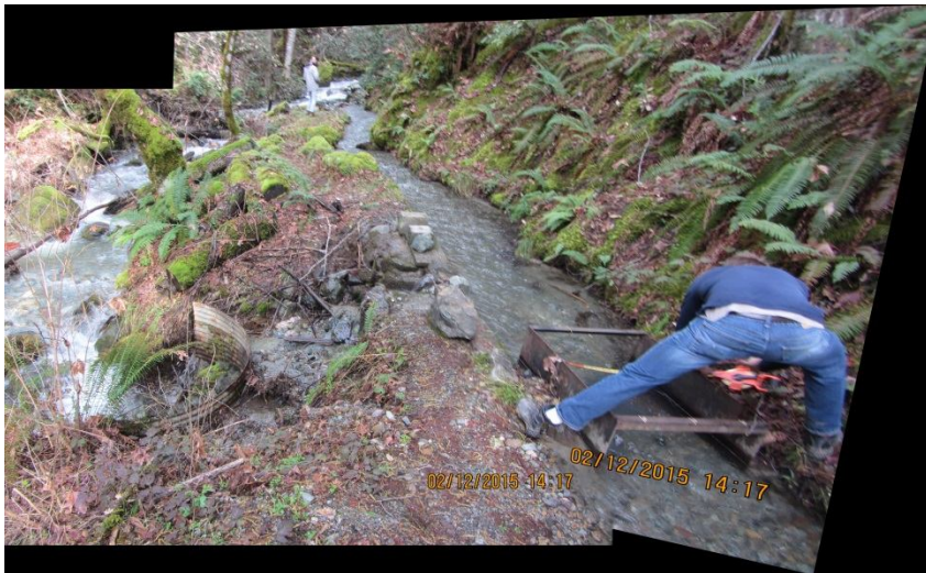
Image 4- shows Point 2, a failure along the outboard berm, approximately 70 feet downstream of Point 1, allowing some of the water in the ditch to flow down to Stanshaw Creek, potentially resulting in erosion and sediment transport. This location appears to have failed repeatedly in the past. The instream flume in the Ditch just downstream of this failure is used to measure flows entering the diversion. (Photo 8454 and 8455)
