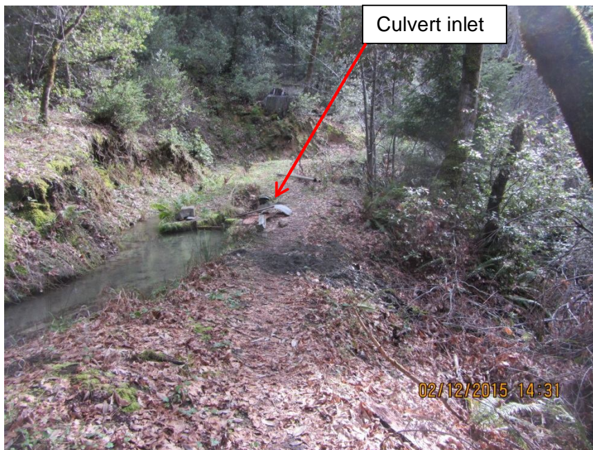
Image 9- at Point 4, shows the partial diversion of the ditch into an unnamed tributary to Stanshaw Creek through the inlet of a 12-inch culvert, before the diversion ditch is routed across the stream in a lined ditch. The culvert is shotgunned, which appears to have caused significant instream erosion in the downslope channel. The stream above the crossing is 3-4 feet wide at bankfull width; the eroded stream channel below the diversion crossing is 12-14 feet wide, and does not appear stable. At this location, I also observed muddy soils in the berm adjacent to the ditch, indicating that seepage from the ditch is saturating surrounding soils, which may lead to catastrophic failure of the ditch. (Photo 8441)
