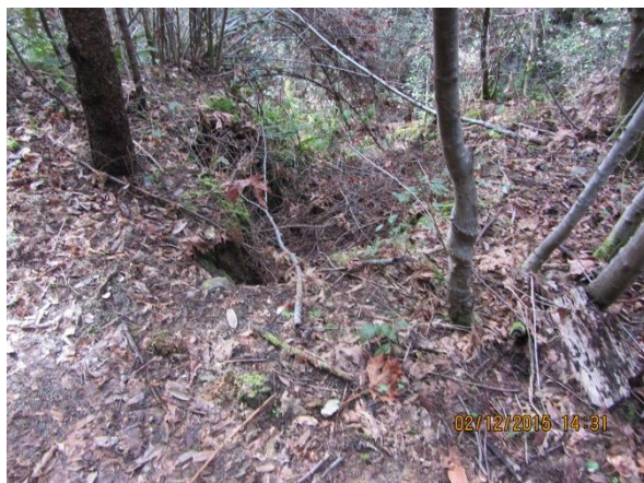
Image 7- shows the erosion channel downslope of Point 3. The void is visible here in the foreground; the erosion extends downslope an unknown distance.
