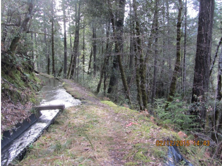
Image 13- point 7, shows the end of the flume in the previous photo; note the black plastic sheeting on the outboard slope face, and the low outboard berm as the diversion ditch exits the flume. The lack of freeboard creates a high potential for overtopping and erosion. The presence of the pipe section and plastic sheeting in the area suggests that the berm or underlying slope in this area has likely failed in the past. (Photo 8483)
