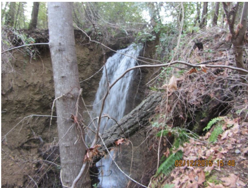
Image 26- Point 20 is the headcut upslope from Irving Creek. This is where tailwater from the Stanshaw Diversion is discharged to an unnamed stream, tributary to Irving Creek. This area is actively eroding. Several trees appear to have fallen recently through erosion of their root masses. I estimate that the headcut erosion has delivered between 1500-2200 yds 3 of sediment to the Irving Creek watershed. (Photo 8529)
