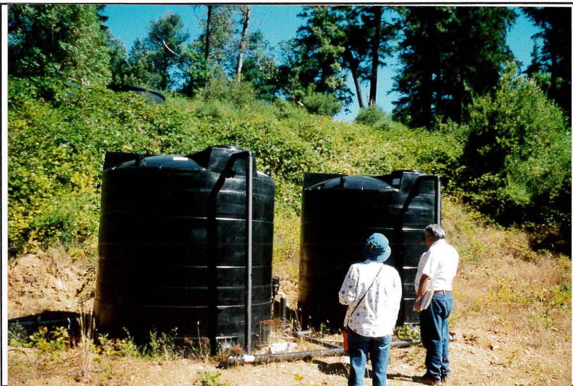
Photo 23. Water purification tanks.
