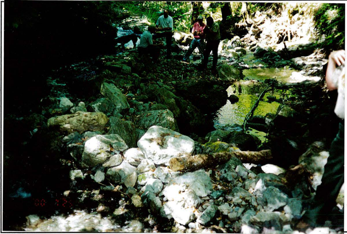
Photo 15. The POD looking downstream. The diversion ditch is on the left. Note the “diversion rocks” in foreground.
