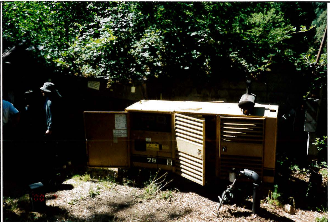
Photo 2. Diesel powered Caterpillar generator
