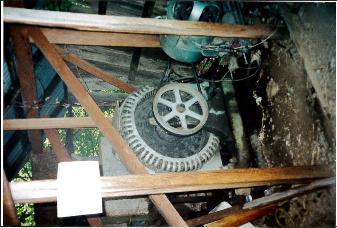
Photo 1. WWII era pelton wheel and hydroelectric generator.
