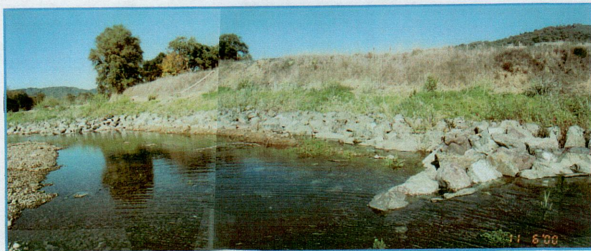
November 6, 2000. View looking upstream of nearly completed construction with willow mattress at river edge and willow clusters above. Note rocks on right of photo.
