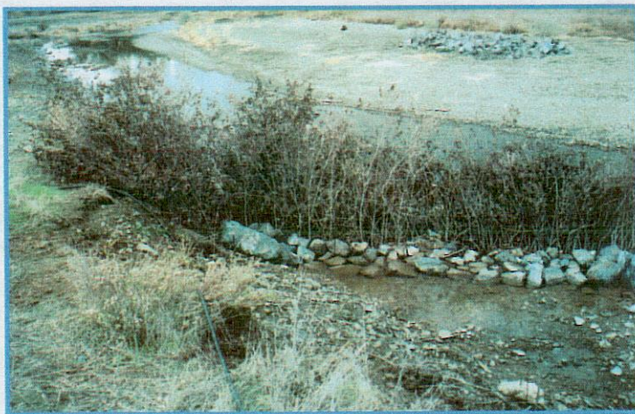
November 11, 1999. Completed willow siltation baffle narrows and deepens channel, and collects sediment upstream of the baffle.
