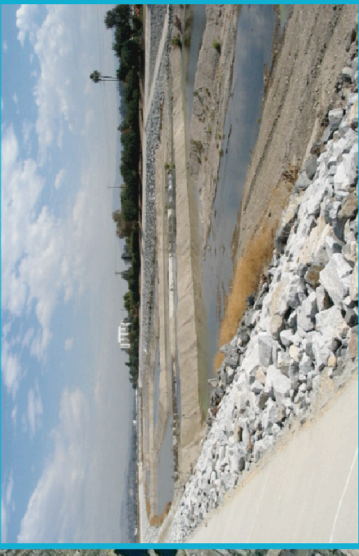
"T" and "L" levees built in recharge section of river near OCWD field headquarters.
