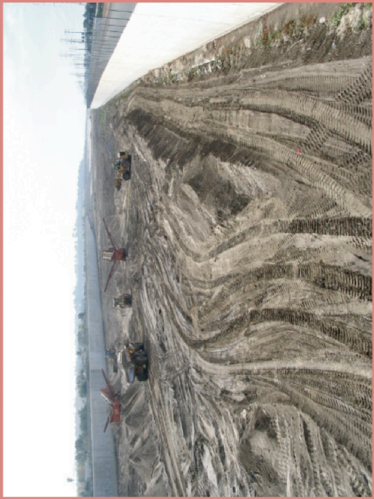
Sand removal by Orange County Flood Control in concrete-lined river channel below Adams Avenue crossing.
