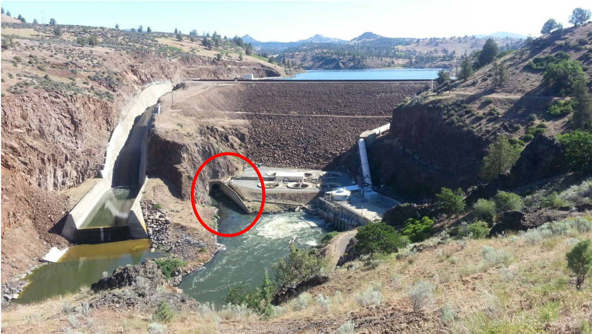
Figure 2: Low Level Outlet Discharge into Klamath River at Base of Iron Gate Dam
