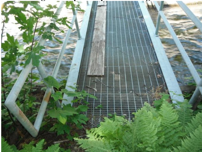
Figure 4. Drum Canal Crossing (GPSID No. YDWMDC037/FS73). Technical Memo 4-2 metadata for crossing notes “planks placed over grate.” Planks do not span the entire length of bridge.
