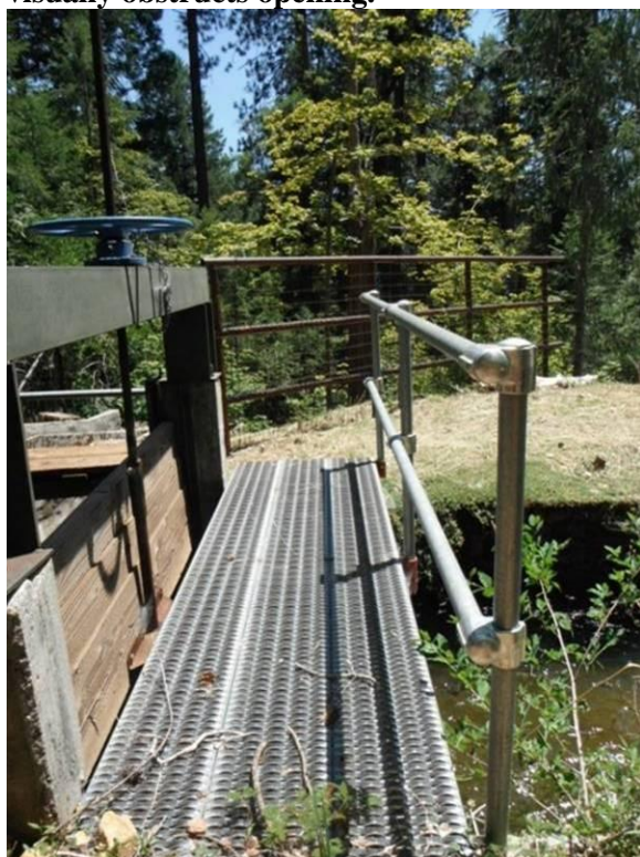
Figure 5. South Yuba Canal (Metadata FSID210; no GPSID). Crossing classified in Technical Memo 4-2 as providing crossing for all species. Crossing is <3 feet wide; fencing on south side visually obstructs opening.
