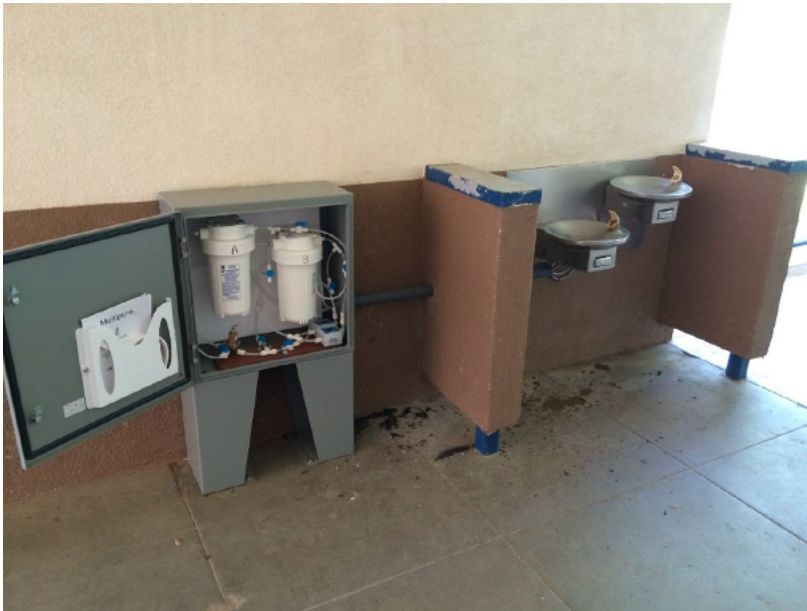
Figure 9. Example Point of Use Treatment Device 19
