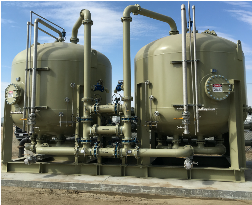
Figure 8. Example of Wellhead Treatment
