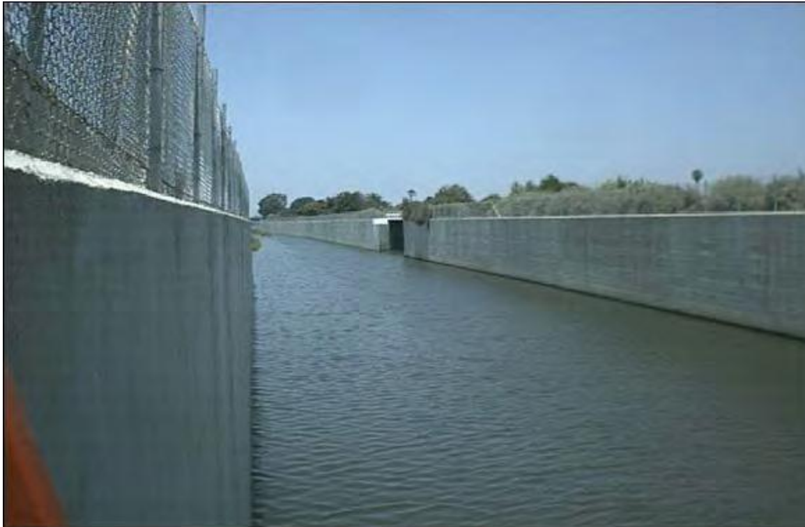
Figure GB-10. Reach 1, Photo REC Survey location, just upstream of inflatable dam. The water behind the dam can be about 1.5 ft. deep. (UAA Analysis GB)
