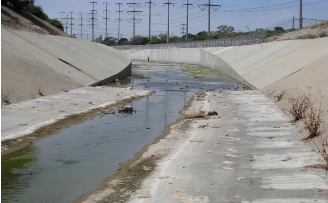
Figures 2-9. Reach .1 Facing downstream, shows transition from vertical to trapezoidal channel. (CDM UAA Technical Report GB)
