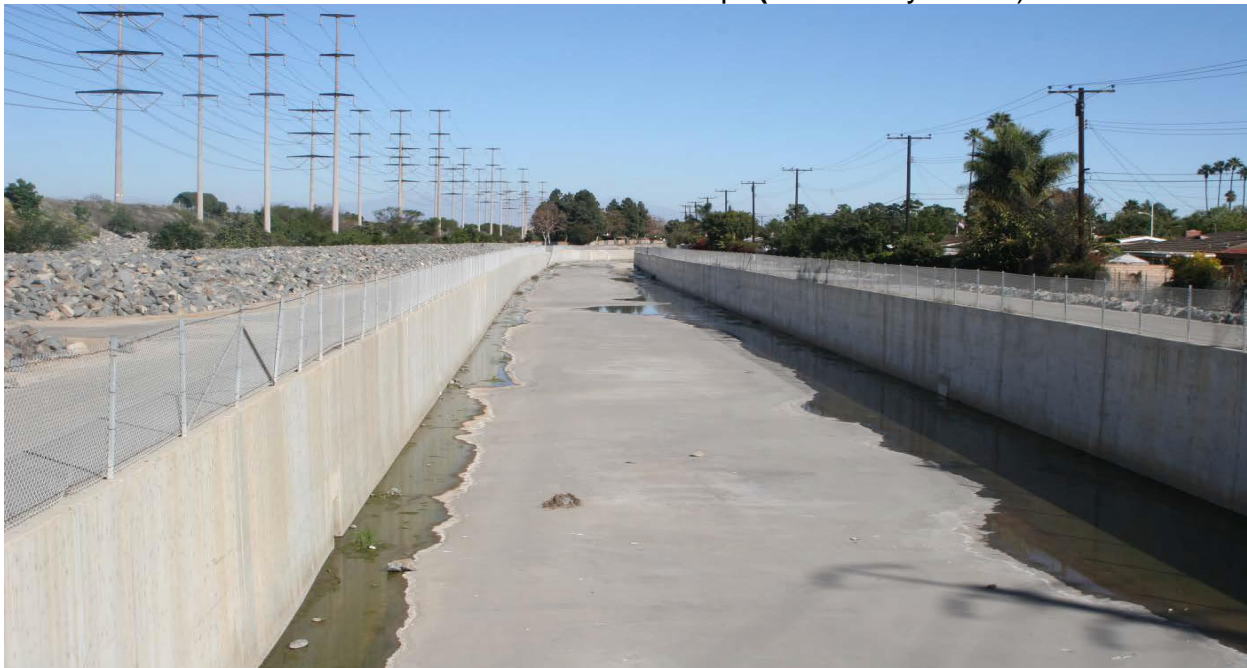
Figure GB-7. Reach 1, facing upstream. REC1 and REC2 uses are not attainable in Reach 1. (UAA Analysis GB)
