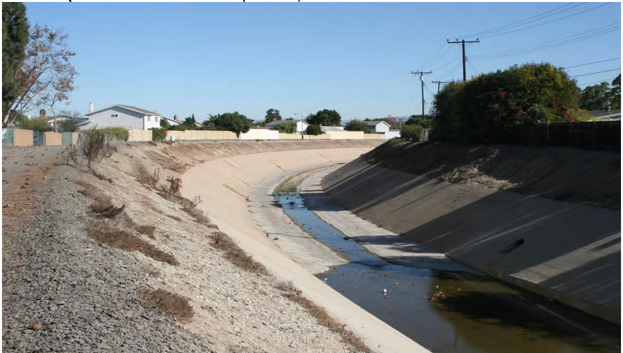
Figure GB-12. Reach 1. Facing upstream, the trapezoidal section is 0.20 mile in length.
