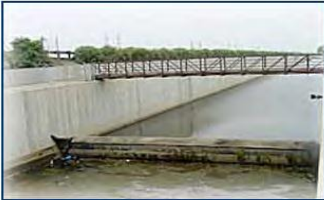
Figure GB-3. Rubber dam diversion at the Greenville-Banning Channel. The dam separates the Tidal Prism Reach from Reach 1. (UAA Analysis GB)
